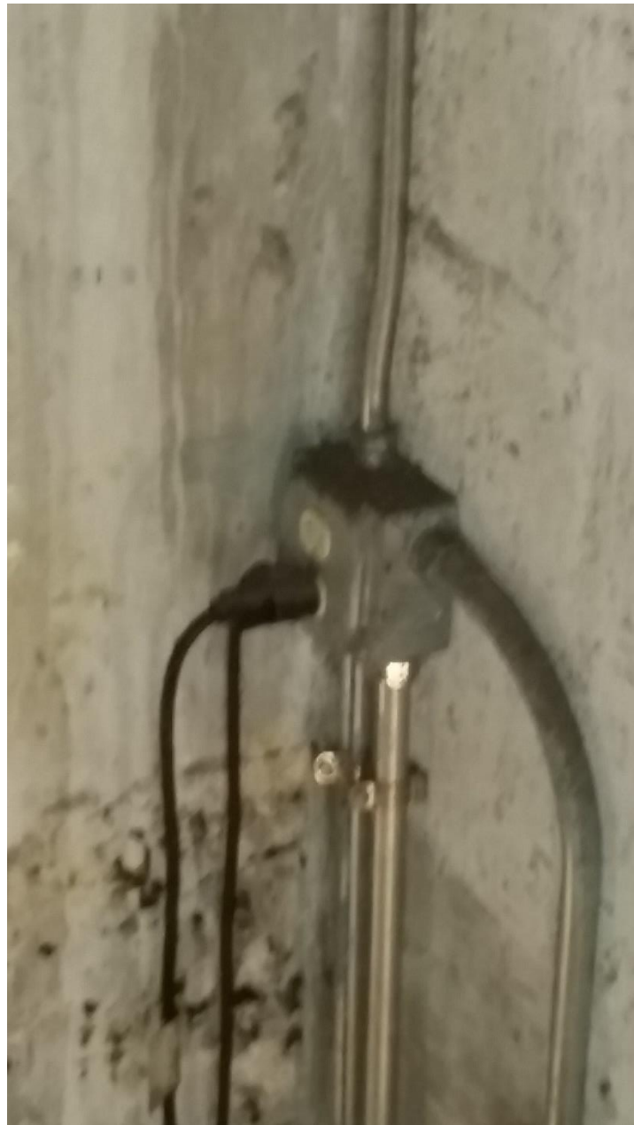
Existing 115vac outlet to sump pump
