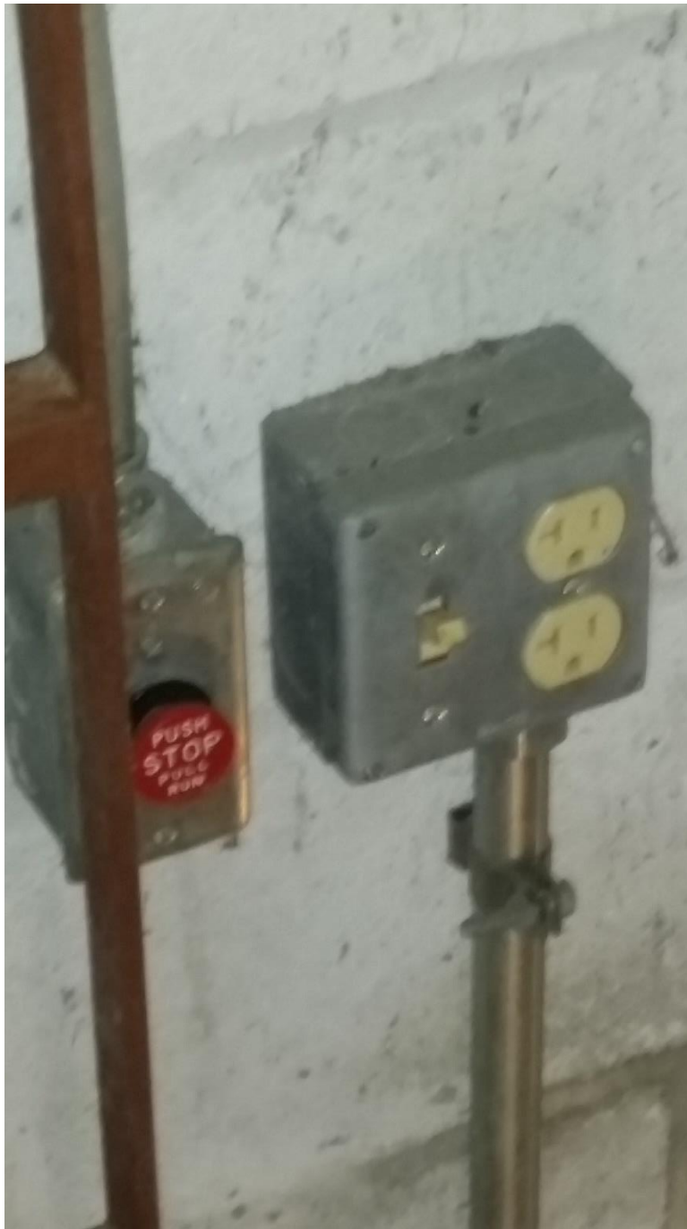
Existing 115vac work outlet on East wall of elevator pit. Scope of Work/RFP--Electrical
